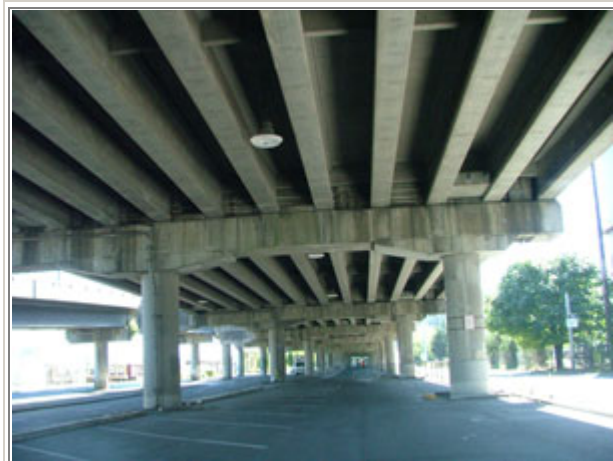
West Seattle Bridge. Use of fly ash in the main deck and silica fume in the bridge deck.
